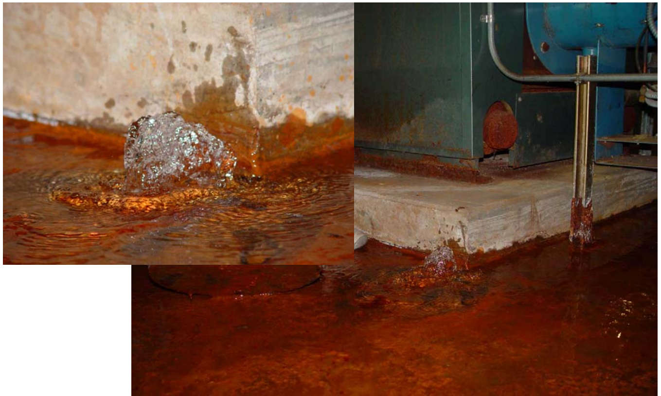
Picture 1.12. Smith basement, showing water damage to boiler (typical)
