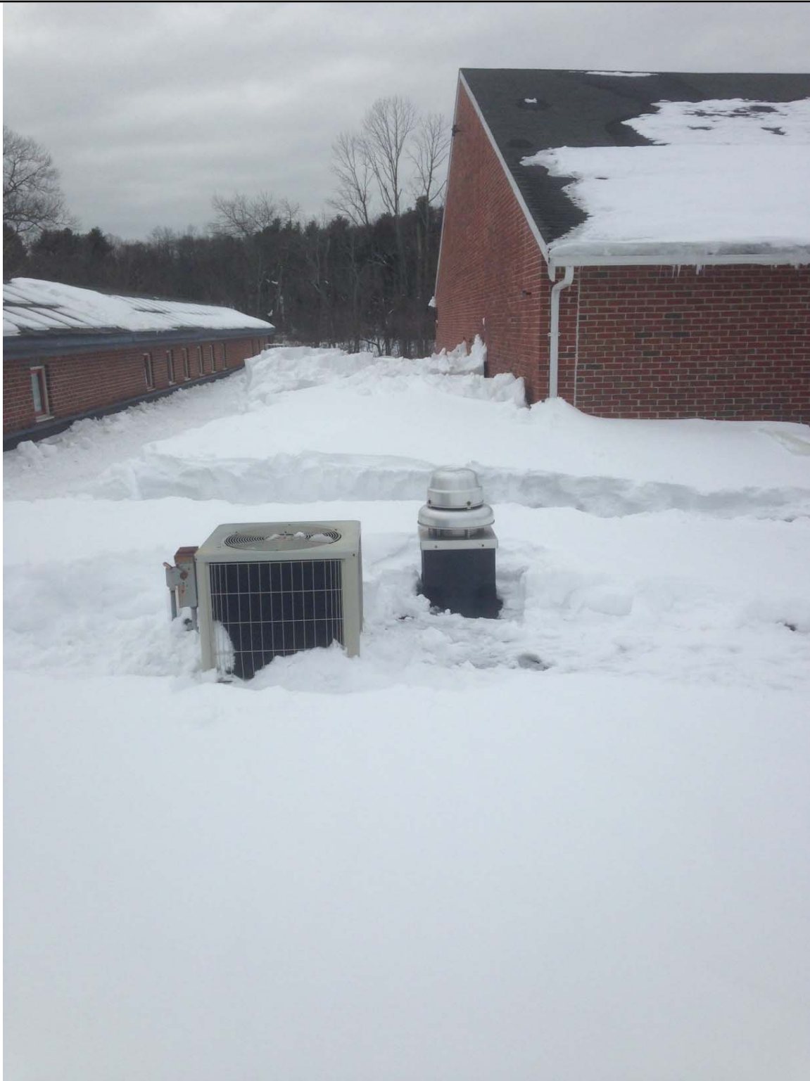
Picture 1.2 Roof were designed before code changes for increased snow loading and drifting, requiring shovelling under certain conditions. Note poor insulation on 1953 section to the left, shown by melted snow.
