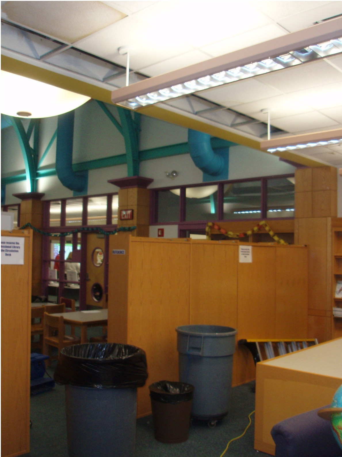
Picture 1.81 Roof leaks under certain conditions impact instruction.
